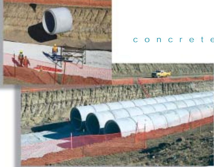
A portion of the storm and sanitary sewer infrastructure for Omaha's waterfront project consists of a triple line of 108-inch diameter RCP.
